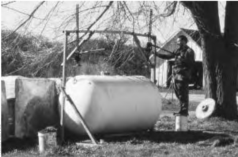
13.13: Tom Blinks uses 2-inch steel grid beam and a pair of jacks to lift a propane tank.
